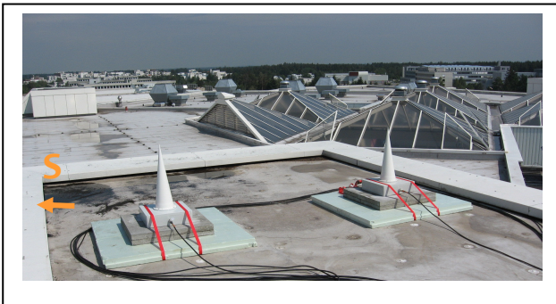
Figure 3 Navigation antennas with omni-directional pattern on EADS-Astrium building
